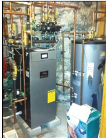
New boiler keeps the Sisters warm at the Medical Missionaries of Mary's home in Somerville
